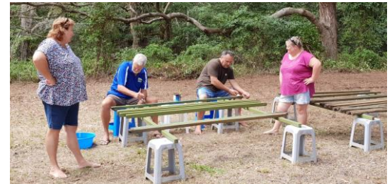
Paul and Shorty painting the rest of the shade shelter poles . . . under supervision!
